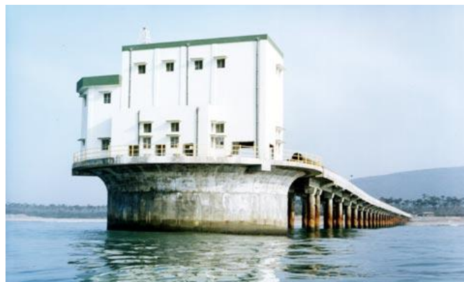
Figure 4: Jetty mounted pipelines
